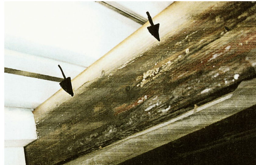
Rotting rafter caused by condensing outdoor humidity
