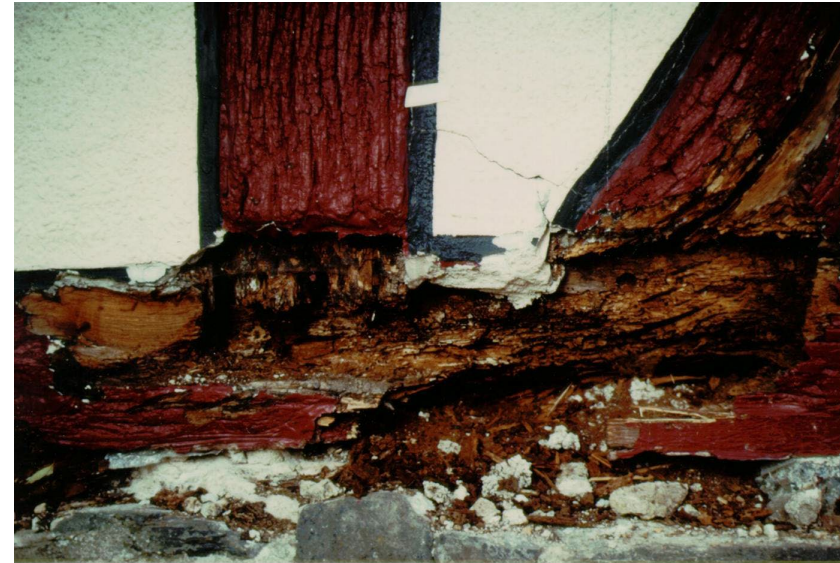
Rotting timber structure caused by driving rain
